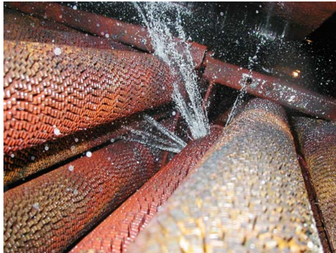
Figure 6 - FAC leak in Tube Mid-Span
