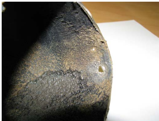
Figure 5 - FAC Damage to Tube interior
