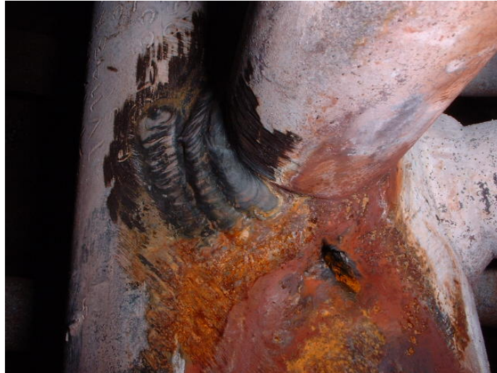
Figure 4 - FAC Damage to Header
